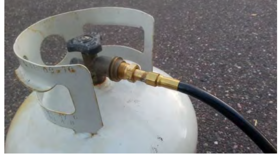
POL Valve on LP Tank
